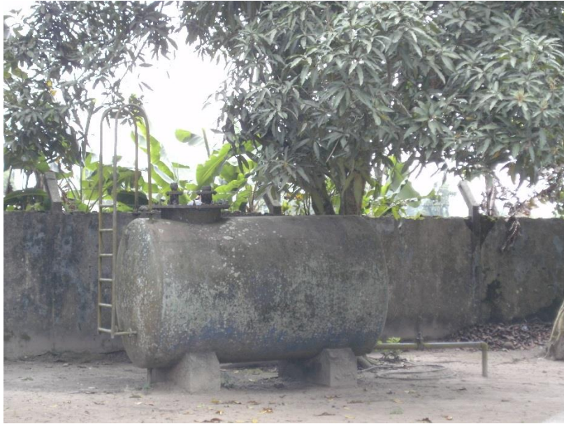
Fig.22: Ughelli North Urban Water Board Division treatment plant.
