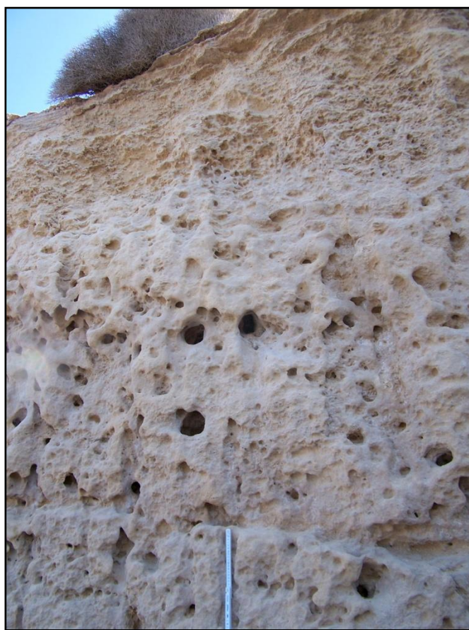
Figure 42: Calcarenite affected by calcretization and honeycomb weathering near Sifnaikos bay
