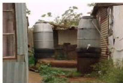
Low-pressure ground tanks supply the water needs of two adjacent households.
