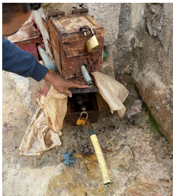
Fig. 22: Two water meters protected by a lock inside of a tannery (Photo: V. Immervoll, Marrakech, February 2024)
