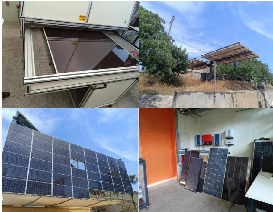
Photo 2. CRES renewable installations and solar research facilities (Photographs by Ektoras Leventis)
