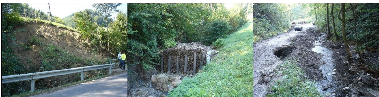
Figure 3: Documented damages of the flood event in 2012 in the Redtenbach Catchment (Source: Wildbach und Lawinenverbauung Ereigniskataster (2012) ).
