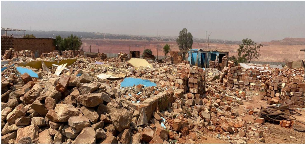
Abbildung 8. A demolished house after eviction by a copper and cobalt mining company in Kolwezi, the Democratic Republic of Congo in September 2022. (Photo by Jean-Mobert Senga/Amnesty International)
