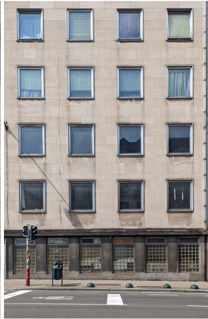
Figure 17. Façade Defacqz. All tilting windows are obstructed by some reused materials. Photo by the author, 2024.
