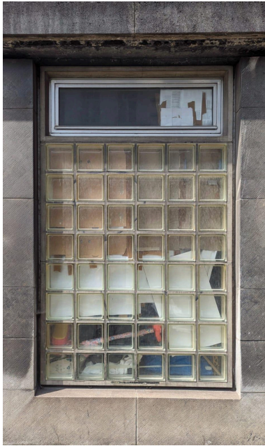
Figure 16. Façade Defacqz. MDF and other materials are visible through the glass bricks. Photo by the author, 2024.
