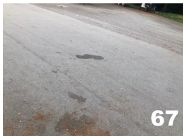
“Too much asphalt”
