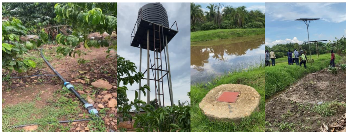
Figure 10. Shows ground irrigation water pipes, a water storage tank, water dam/reservoir, underground water pump and solar panels to power the system.
