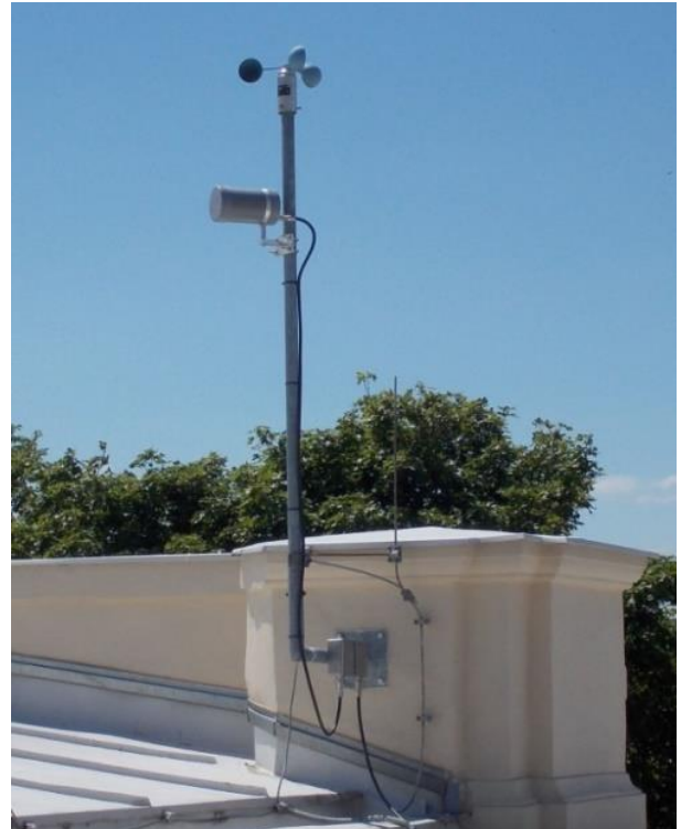
Figure 39: Directional antenna and frontend amplifier mounted at the roof of the IfA building
