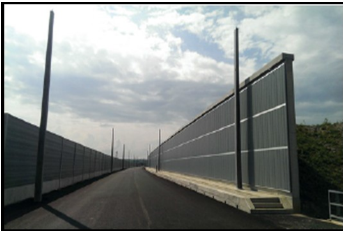
Fig. 20 the noise barriers: picture by ÖBB Infrastructure
