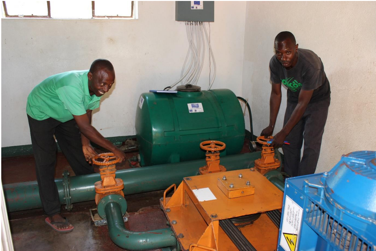
Figure 7: Three Jet Pelton Turbine with power house workers opening the jets
