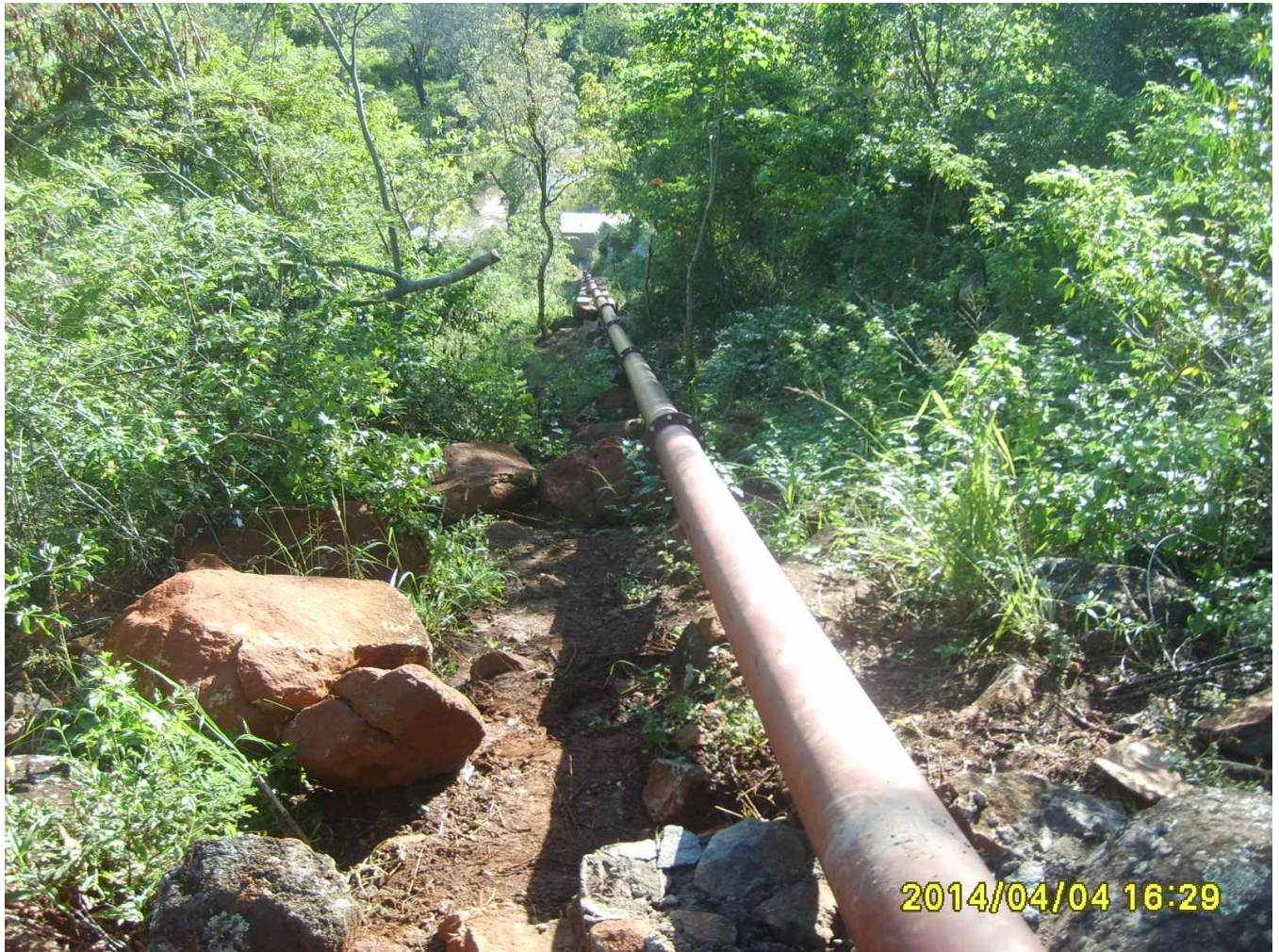
Figure 11: The penstock, (head) caring water to the turbine house
