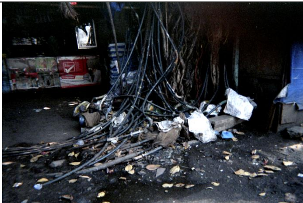
Figure 101: Bunch of water connections with motors hidden under the plastic bags.
