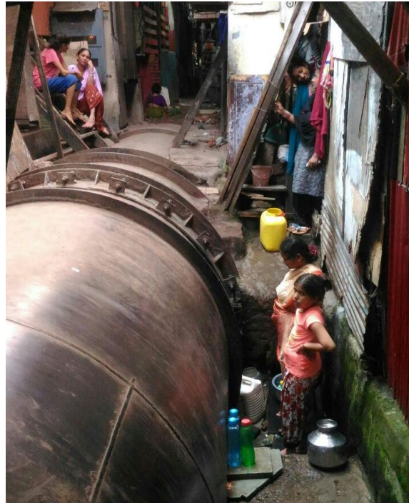
Figure 11: A woman and a girl are fetching water from the leakage in the pipeline.
