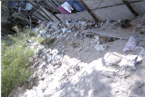
Figure 58: Illegal water pipelines leading to individual households.
