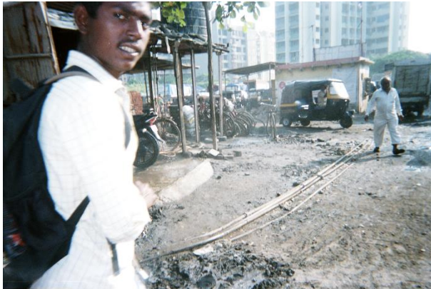
Figure 16: Official overhead water pipeline that passes through Ambujwadi.
