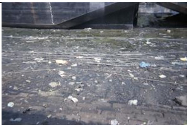
Figure 116: Illegally extended over ground water pipelines at the creek.
