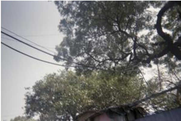
Figure 83: Illegally extended over ground water pipelines.
