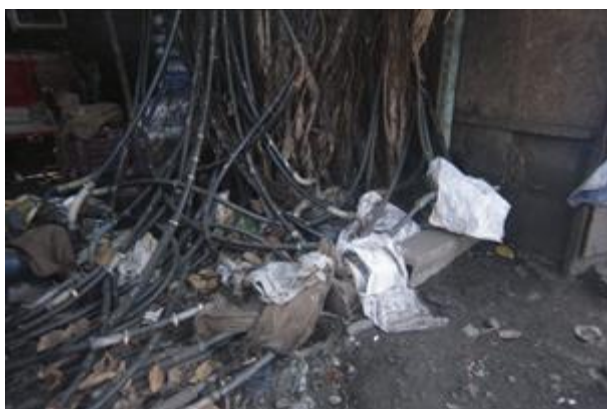
Figure 128: Bunch of unofficial water pipelines. Plastic bags are used to camouflage the motors.
