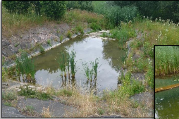
Figure 41. Retention basin (AW04). Although it is completely man-made, a sandy ground has been deposited and grass-like vegetation is growing. (© HÖRWEG)
