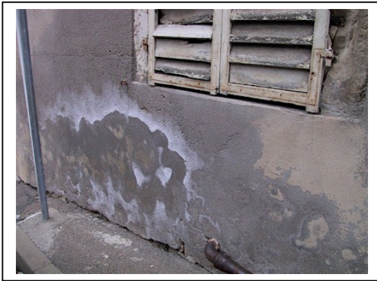
Fig.63, salt damage to buildings, photo by author, 2007
