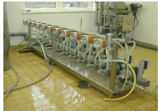
Fig. 15: Hydro-cyclone plant (ZFT, 2007)
